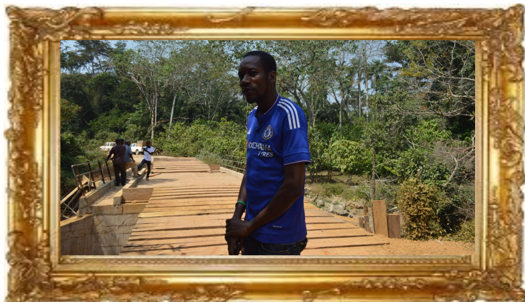
Kailahun DPCU Project Engineer on supervision at one of the Project constructed bridges in Kailahun District
